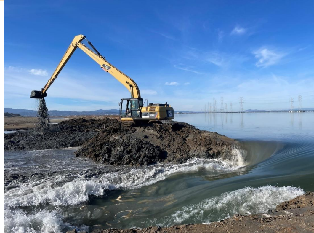
Levee breach at South Bay Salt Ponds. Photo: South Bay Salt Ponds Restoration Project
